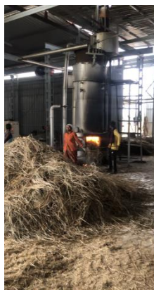
Steam Generator Fuel
